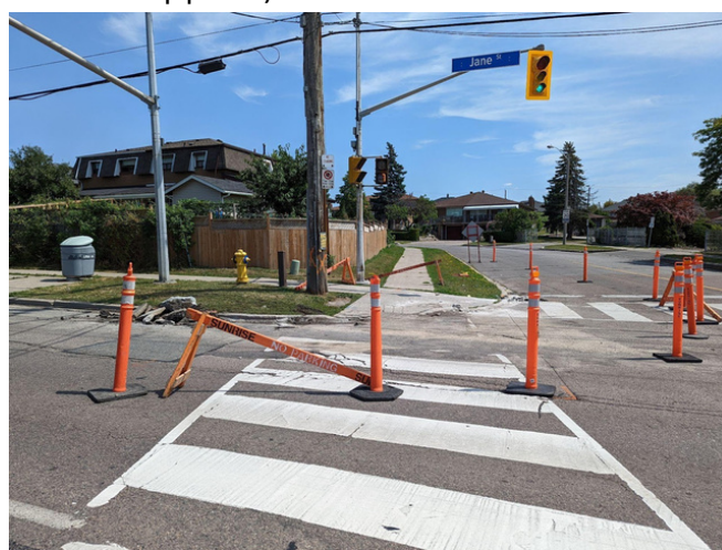
Image 7: A second photo of the construction pylons blocking the pedestrian crossing at Jane Street and Rita Drive.
