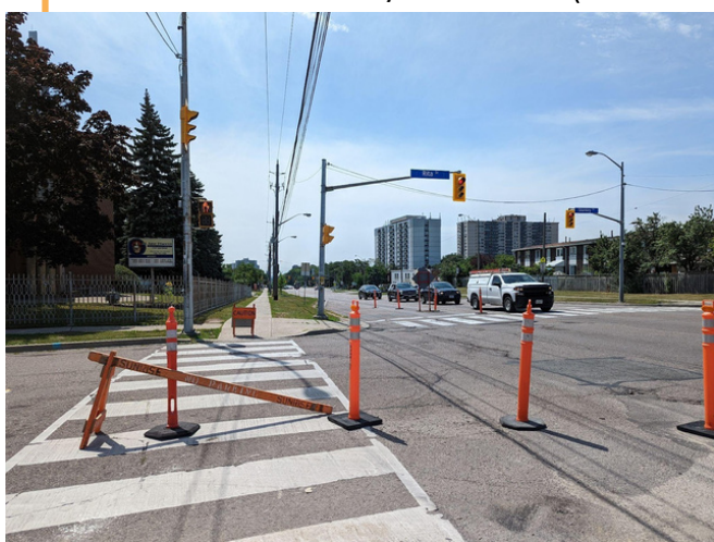
Image 6: Construction pylons block the pedestrian crossing at Jane Street and Rita Drive, pushing residents to walk in the road or on the other side of the street.
